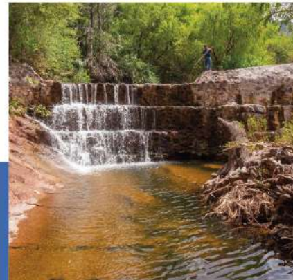
Fig. 3. A small rural dyke delivers water for nature, agriculture and the households. © Pablo Herrerías Guerra.
