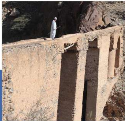
Fig. 1. Canal-bridge to allow water overtaking a depression in a valley ( wadi bari kharous ). © University of Nizwa.
