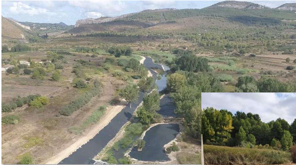
Riverbank restoration work on the river Albaida, in the municipality of Bellús
